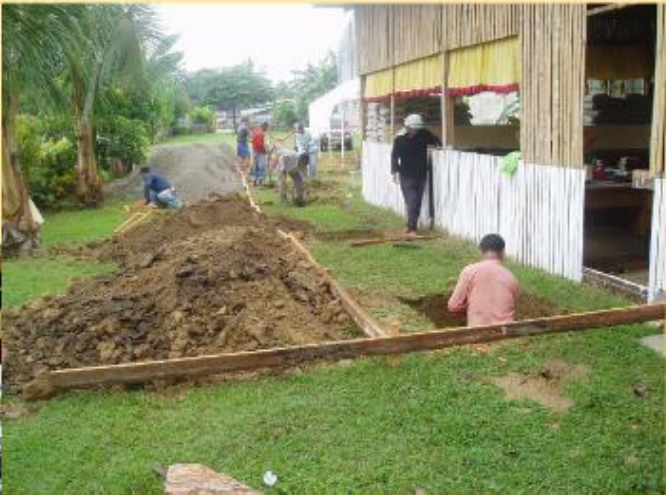
Church volunteer workers digging the holes for the post foundation. At the back in blue shirt Pastor Heber Bartolaba of Jimenez church is cutting wood.
